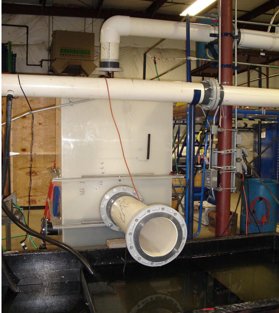
Figure A-2: View showing Up-Flo™ Filter overhead Inlet Pipe, Outlet Pipe and Collection Basin
